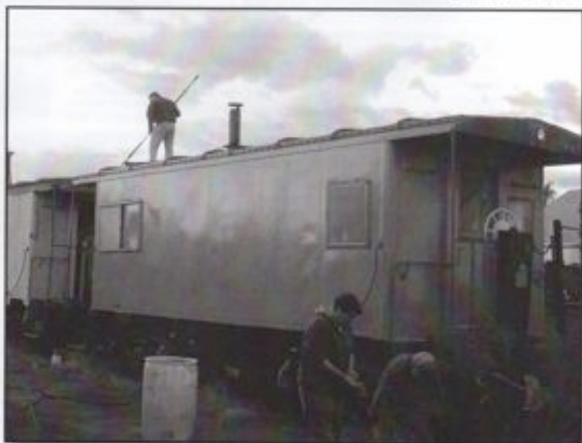
At the top left John Thompson (on roof), Paul Strubeck, and Rich Gordard continue to work on C-60.
