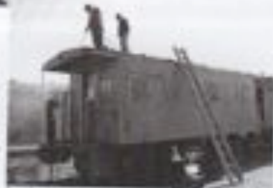
Paul Struback and John Thompson power wash paint off the roof. Photo: Rich Goodhart
